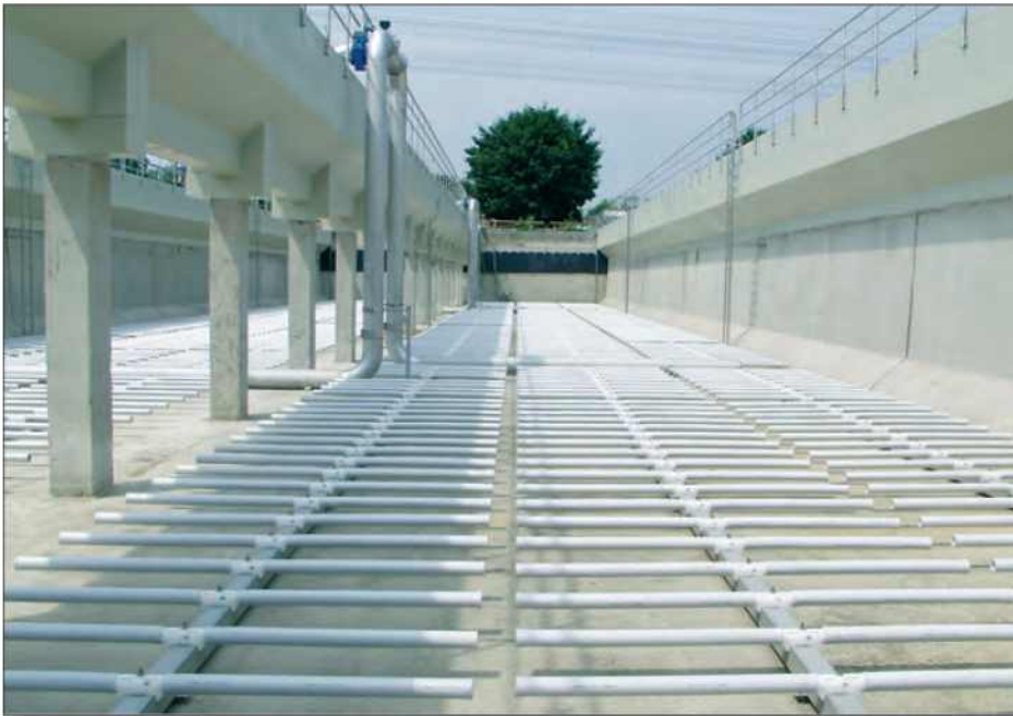
Waste water treatment plant with MAGNUM® 2000 FLEXSIL® membrane tube diffusers.
